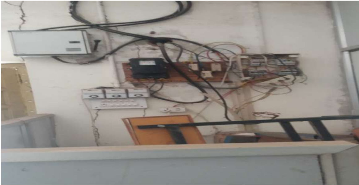
Maintenance of Electrical Infrastructure
